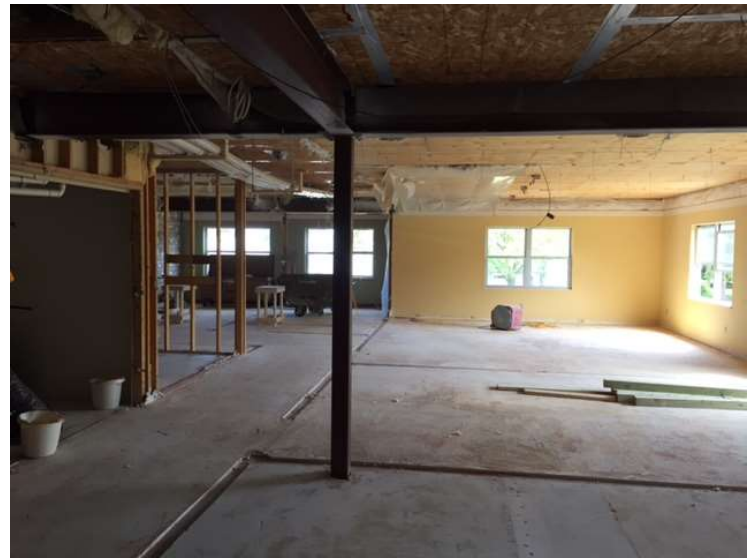
Level 1 demolition is nearing completion. All walls, ceiling, and floor have been removed from site.
