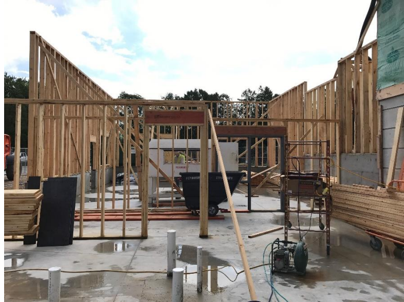
Interior walls are framed for the preschool and braced until the floor trusses are set on the walls and secure.
