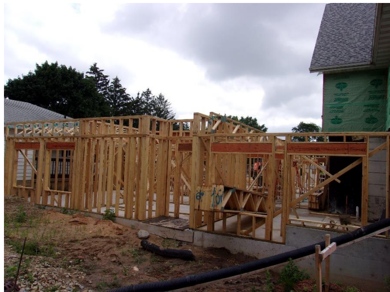
View of the entrance to the preschool from Main Street. Exterior walls are framed and level 1 floor trusses are set. Next to be installed is exterior sheathing.
