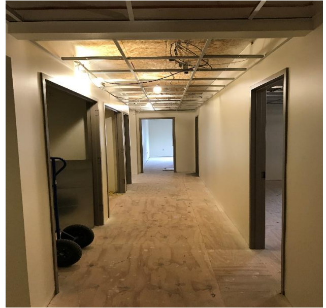
Hallway on 1 st floor. Once above ceiling inspection is complete flooring will be installed.
